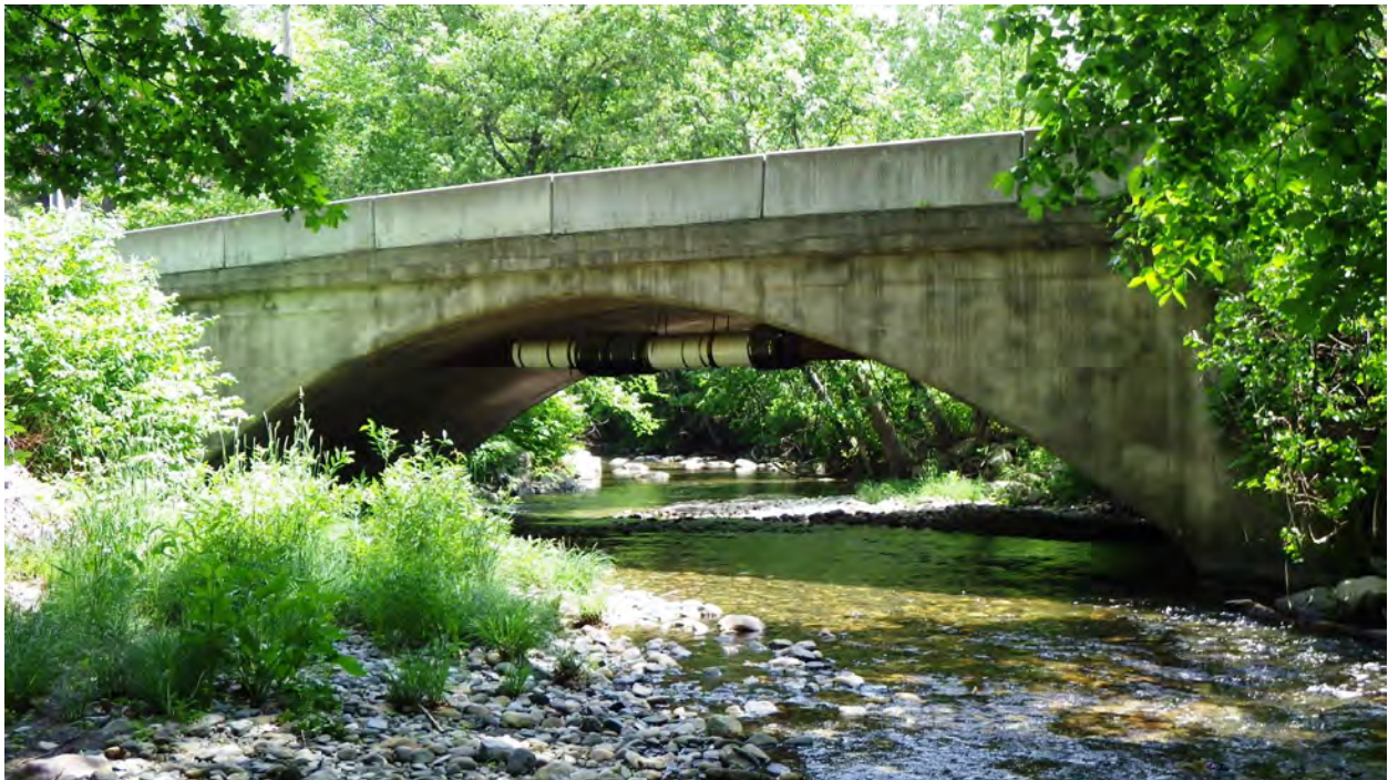
Figure 3.4 Looking upstream at bridge; note cobbles in streambed and utility pipe on underside of bridge. [Inspection photo dated 2015]
