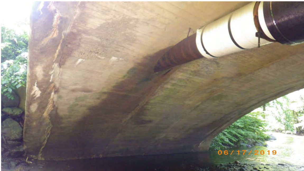
Picture 9: Arch Ring – Note cracking, seepage and efflorescence at fascia and seepage at the embedded waterline
