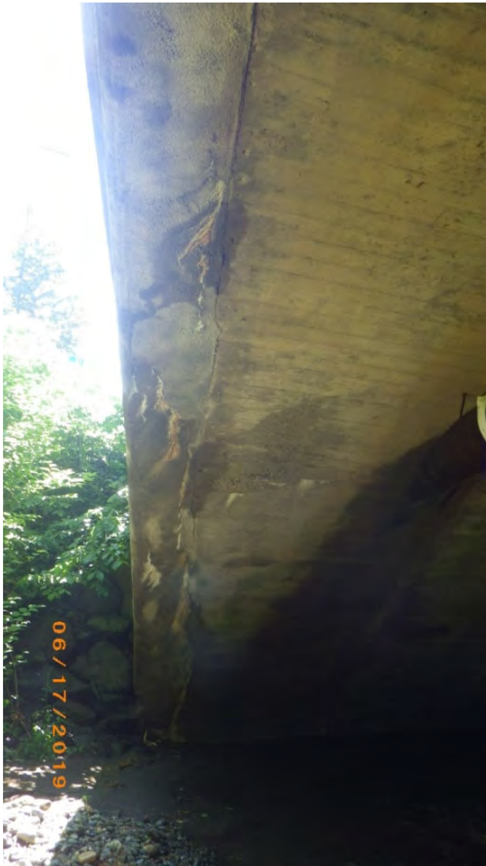
Picture 11: Barrel of the arch - note scattered fine longitudinal and map cracks below the fascia areas with efflorescence staining
