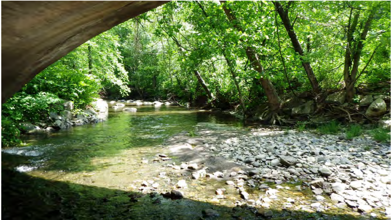
Figure 3.3 Looking downstream from underneath bridge; note cobbles and boulders in streambed and along embankments. [Inspection photo dated 2015]
