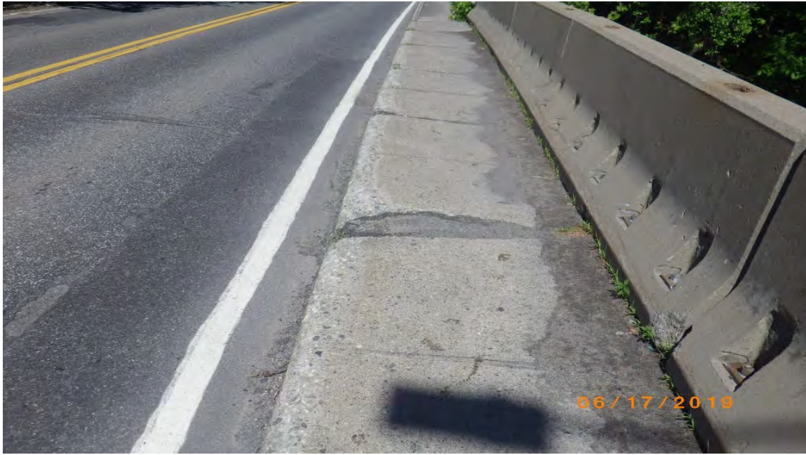
Picture 6: Poor Sidewalk Condition
