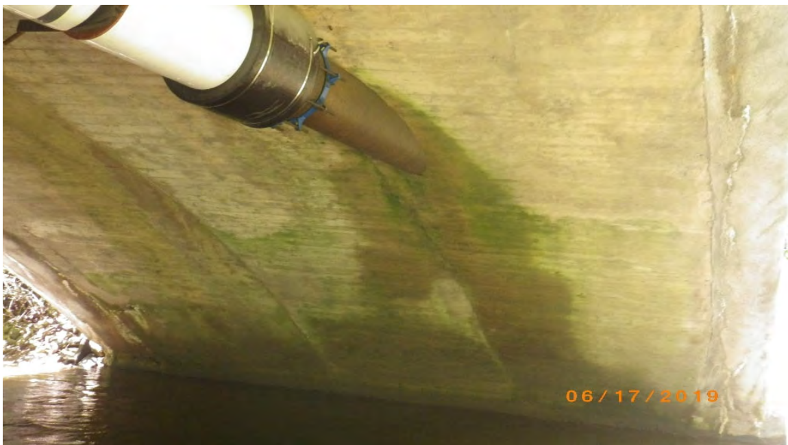
Picture 10: Arch Ring – Note cracking, seepage and efflorescence at fascia and seepage at the embedded waterline
